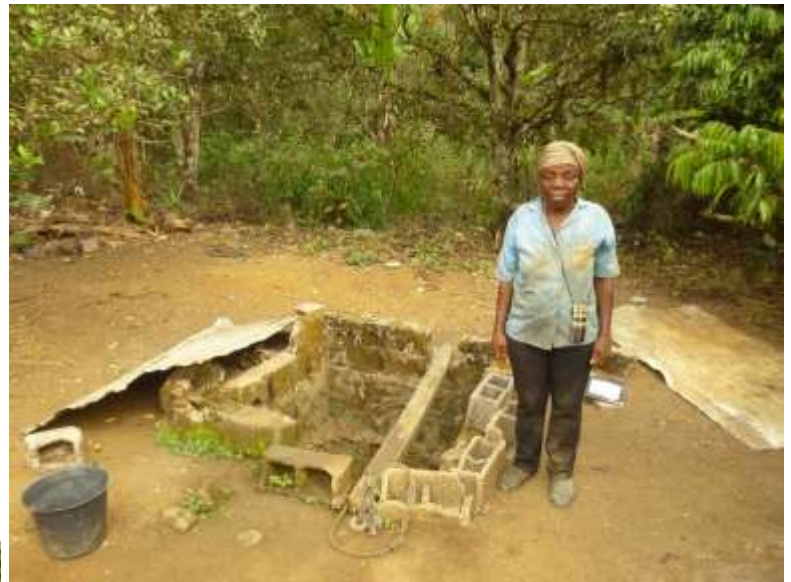
Figure 5. Very basic well. Often villagers will begin construction before they have all the money, so wells will look like this until they can afford to add a concrete skirt and cover.
